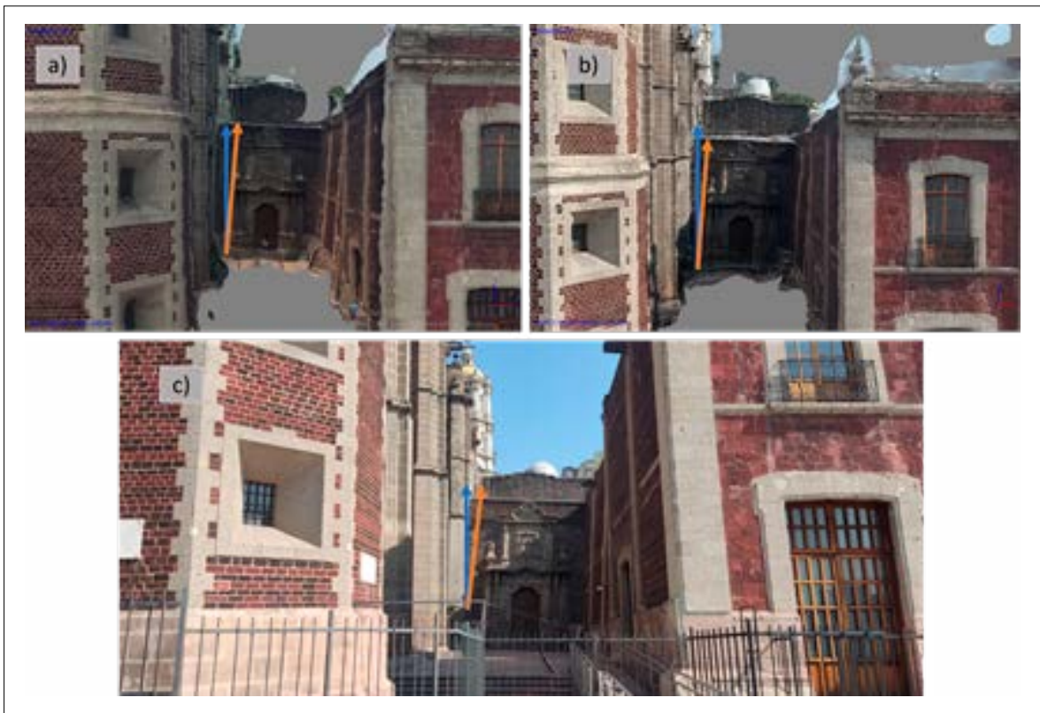
Figure 7. Representation of the property tilt (red line) relative to a vertical reference (blue line). Best 3D models: PL1 (a) and PL2 (b); bottom: actual view of the property (c).
