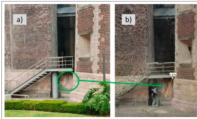
Figure 13. Fracture between the Old Basilica of Guadalupe and the adjacent museum at the rear of the property. a) Field photograph showing the fracture; b) Image extracted from the 3D model.
